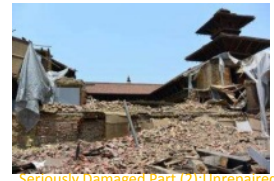
Seriously Damaged Part (2):Unrepaired part
