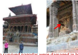
Even survived pagodas were damaged in brick
