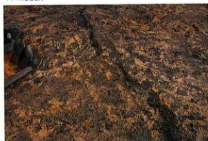
H-40 床面地割れ痕
