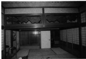
間仕切欄間切抜き三扇左端扇欠損
