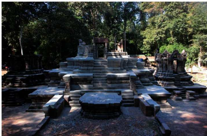
Fig. 28 View of the reassembled platform and façade of the central sanctuary (view from the east)
