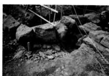
B・C面入隅部根石の飼い石と裏込めは築城時か
