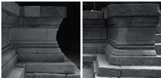
Fig. 40: South stairways of the Central Sanctuary after restoration (Left: west side, Right: south side)
