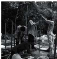
Photo 21: Quality inspection by a simple penetration test immediately after completion of the test foundation
