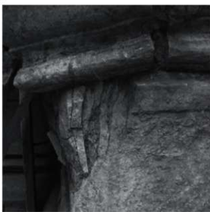
Fig. 39: Damage to a stone panel
