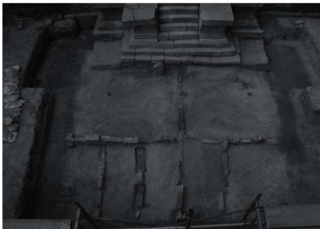
Fig. 53: Digging work and the stone lines in the foundation (viewed from the south)
