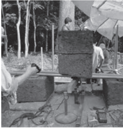
Photo 22: Quality inspection by a loading test immediately after completion of the test foundation
