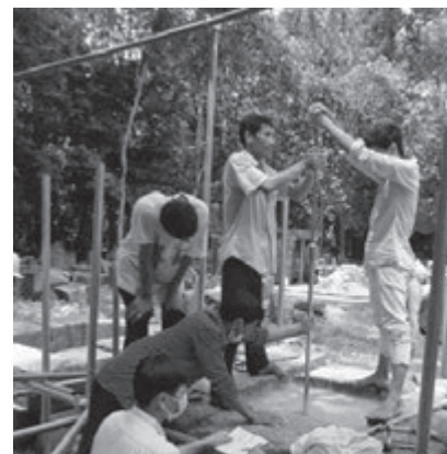
Photo 21: Quality inspection by a simple penetration test immediately after completion of the test foundation
