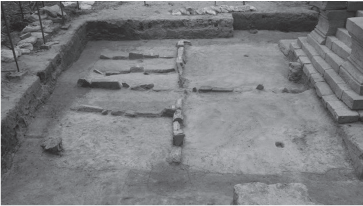
Fig. 54: Digging work and the stone lines in the foundation (viewed from the east)
